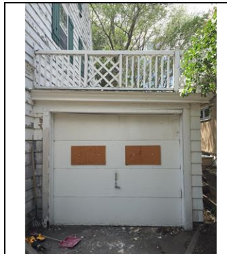
Above: The garage on the north side of the house that will be demolished. 09/12/2019
